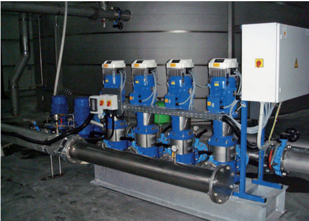
Figure 4 Pressure booster system for pure water supply
