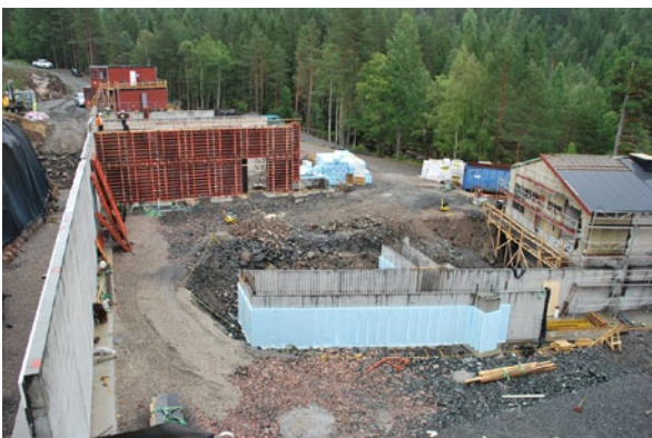
Figure 2. New water treatment works with existing power house. © Source Sweco
