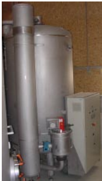
Fig. 4: Compact drinking water unit with control cabinet and ozone generator module
