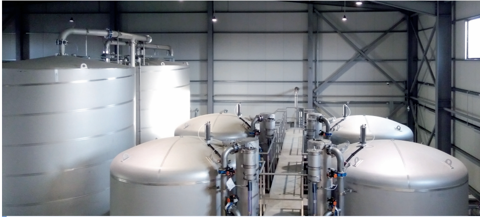
Raw water tank (left) and water treatment (right)
