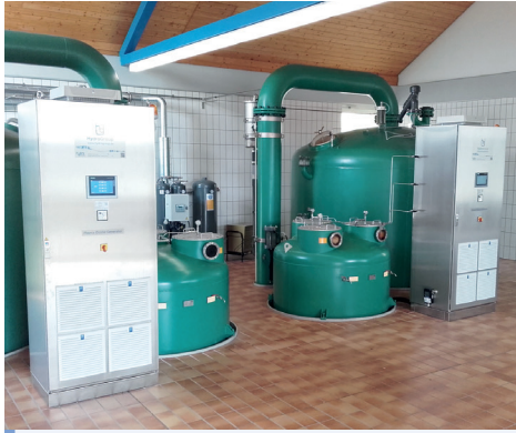
New ozone technology in a waterworks
